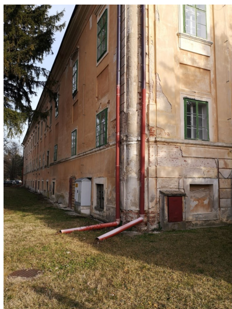
Fig. 3: Damaged corners of the mansion as a result of the original damaged rainwater downpipes (author's archive)
