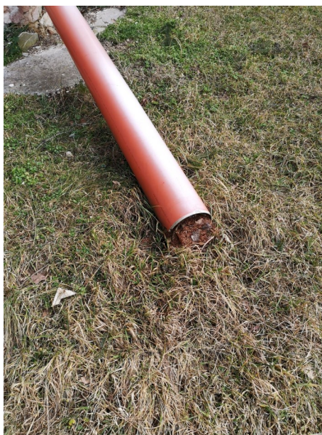
Fig. 4: Neglected Rainwater Maintenance (author's archive)
